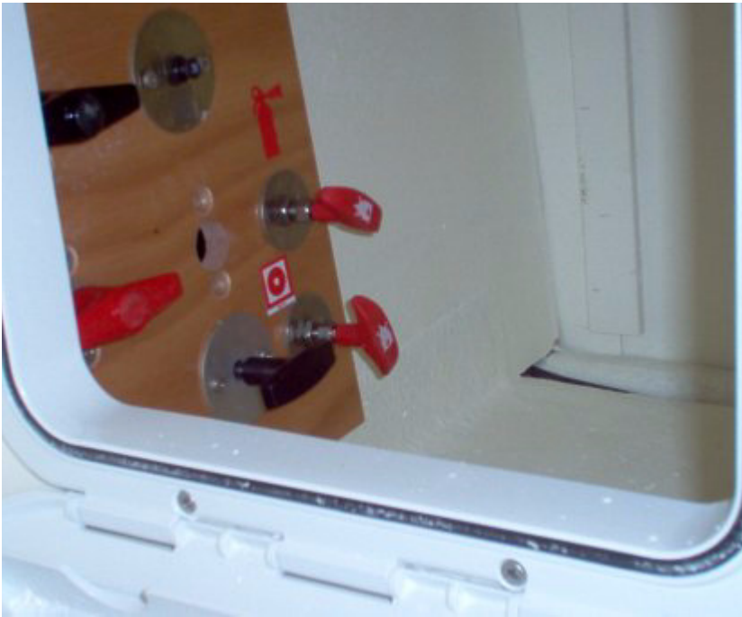
Engine battery switch
